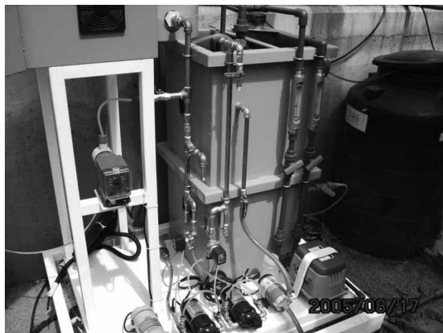
Figure 2. Photos of the MBR pilot plant (from left to right: PLC controller, membrane tank and influent tank).
